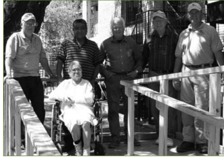
The ramp constructed by volunteers with the Texas Ramp Project will allow Garcia greater independence outside her home.
